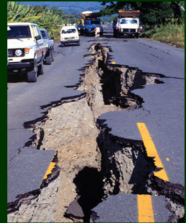
Road destroyed by the Limón earthquake, 1991
